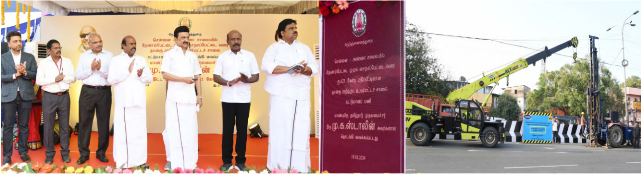
Hon'ble Chief Minister laid Foundation stone for the Construction of Elevated Corridor from Teynampet - Saidapet at Anna Salai, Chennai on 19.1.2024.
